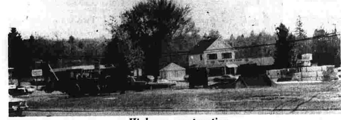
Construction crews have moved into the Vernon Circle and Talcottville areas preparing for changes to be made in connection with the expansion of Interstate 86. The crews are now putting in underground utility wires. Further down they are clearing the area for new ramps to the highway. (Herald photo by Richmond)
